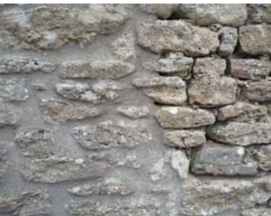
Inappropriate cement pointing to traditional historic boundary wall
